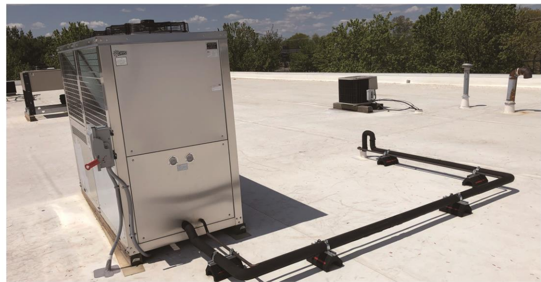
# Roof top unit
